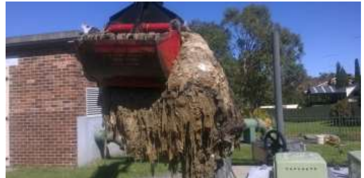
IMAGE: LARGE BUILD-UP OF WIPES EXTRACTED FROM DRAINS SOURCE: https://watersource.awa.asn.au/business/assets-and-operations/court-finds-kleenex-flushable-wipes-not-misleading/
