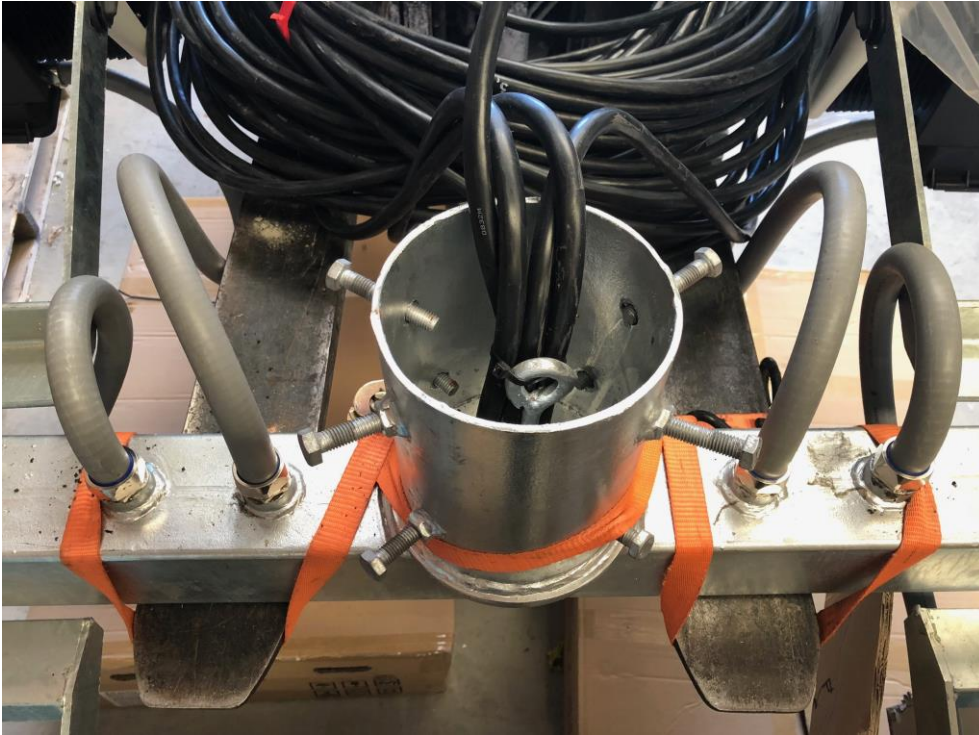
Example of headframe detail with glanded Adaptor Flex and cable support. This also shows the 8-core ELV cabling run from the remote gear trays to the fittings.
